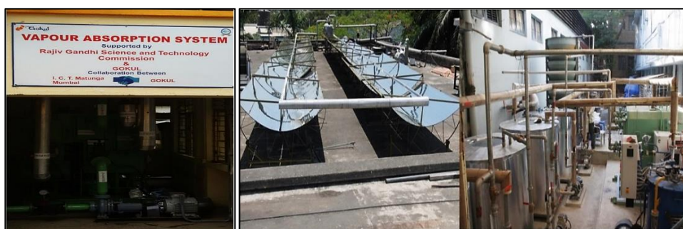
Cold storage facility and set up
